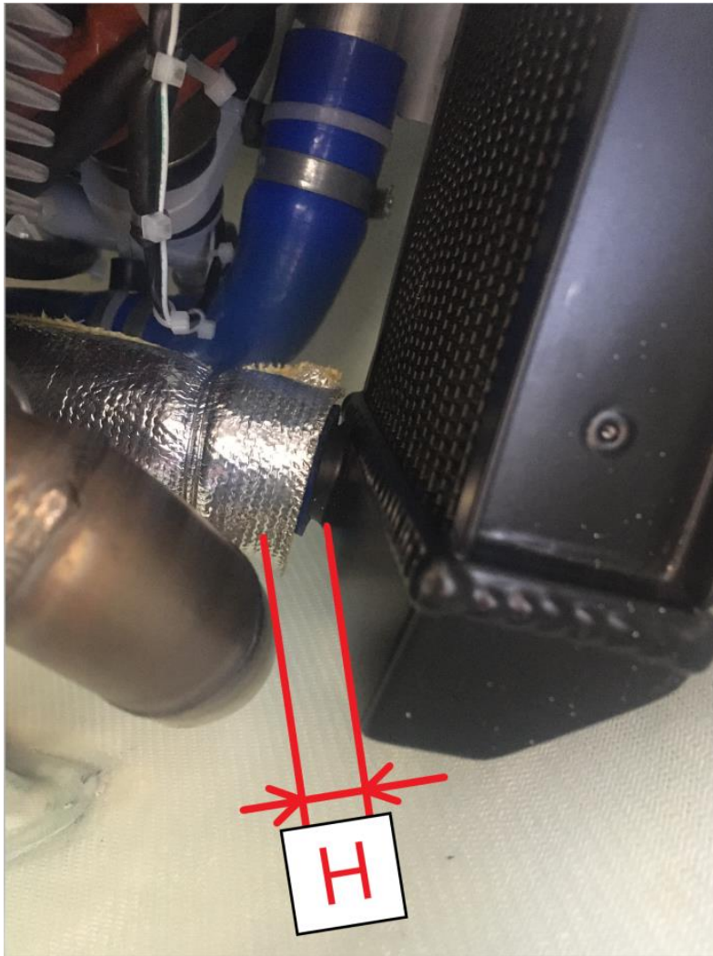
Figure 8: Distance between cooler and exhaust
