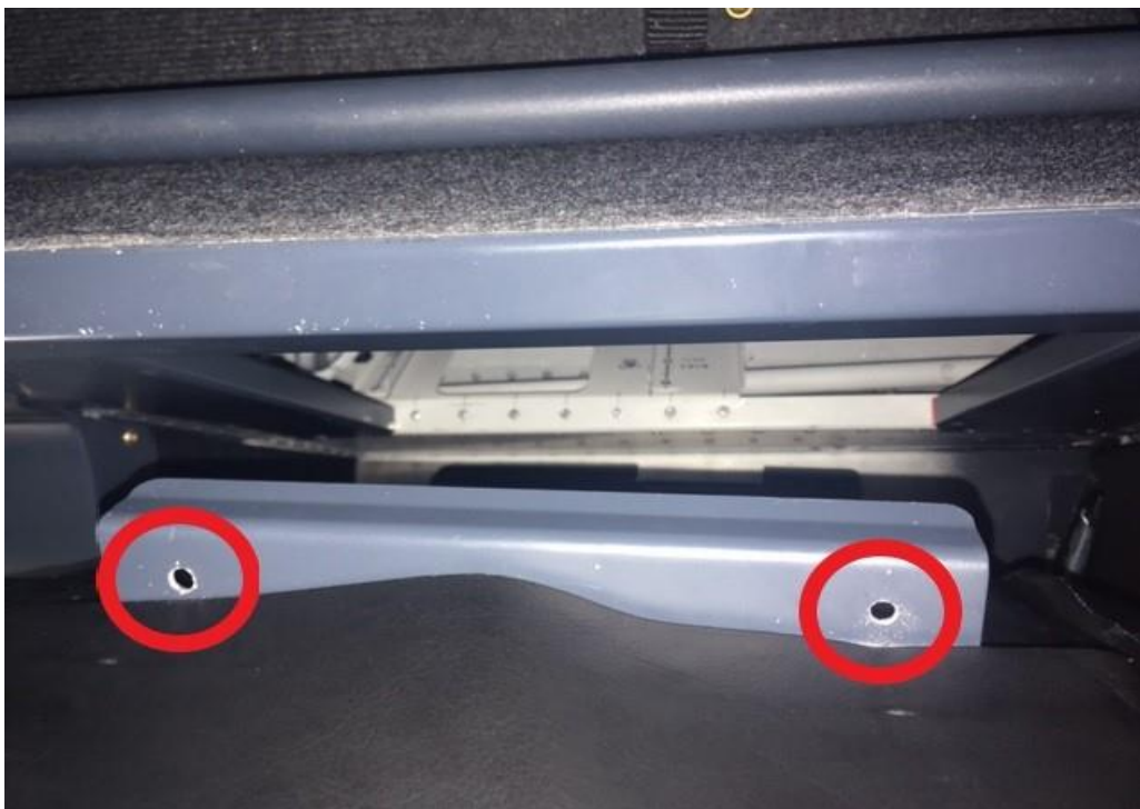
Fig. 8: Holes in the upper locker (attachment)
