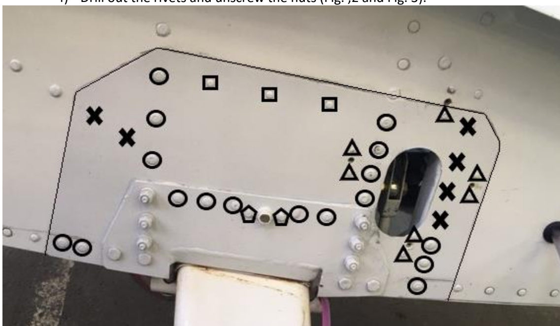
Fig. 2: Main gear attachment patch (left side)
