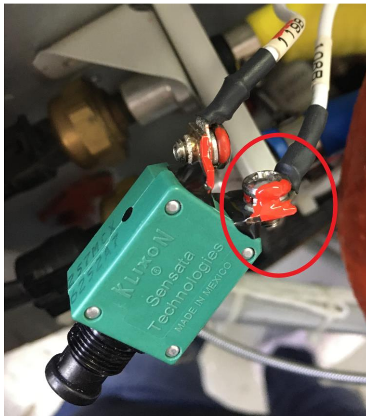
Fig. 16: Fuse secure point
